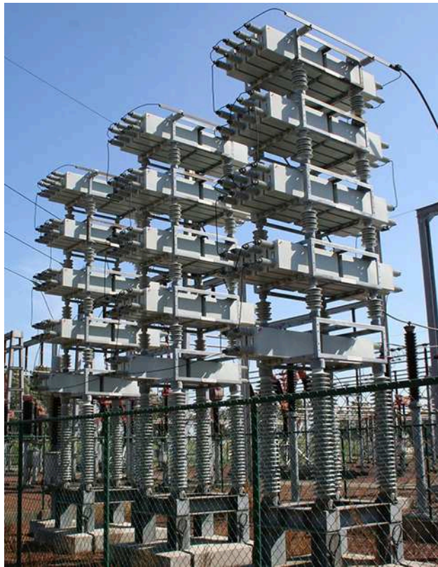
Figure 15.14 Power capacitors are used to balance the impedance of the effective inductance in transmission lines.
