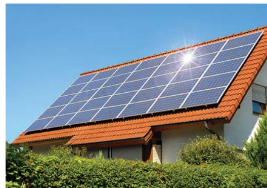
▲ Figure 12 A domestic photovoltaic panel system.
